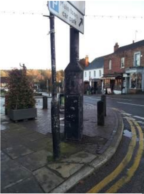
Street furniture in need of maintenance
